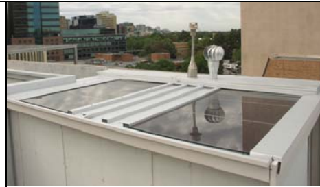
BIPV in the enclosure roof
