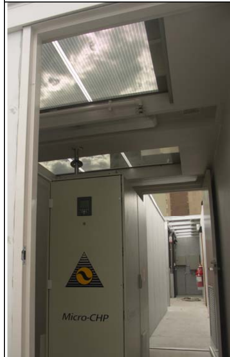
Inside the enclosure showing the fuel cell & the natural light from the BIPV
