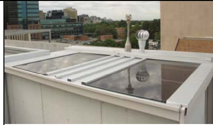
BIPV in the enclosure roof
