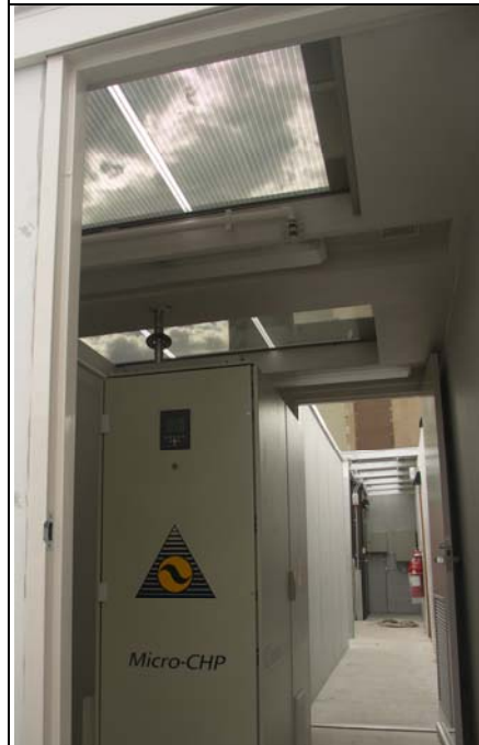
Inside the enclosure showing the fuel cell & the natural light from the BIPV
