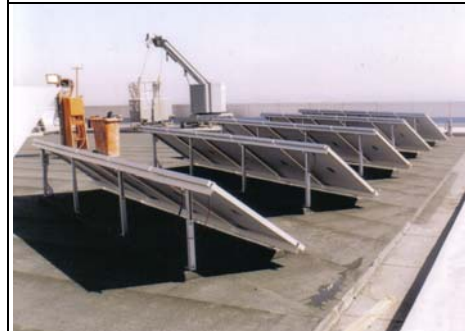
PV panels on the roof showing mounting frames
