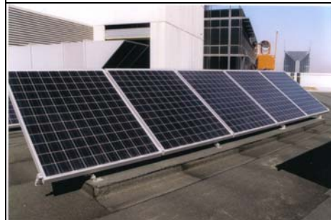
PV panels on the roof (detail)
