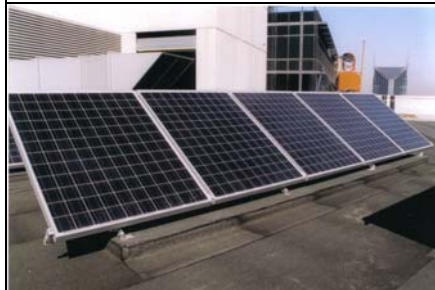
PV panels on the roof (detail)
