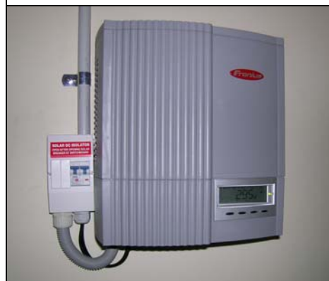
Inverter (located inside the building)
