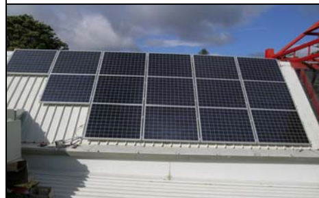
Photovoltaic panels on the roof
