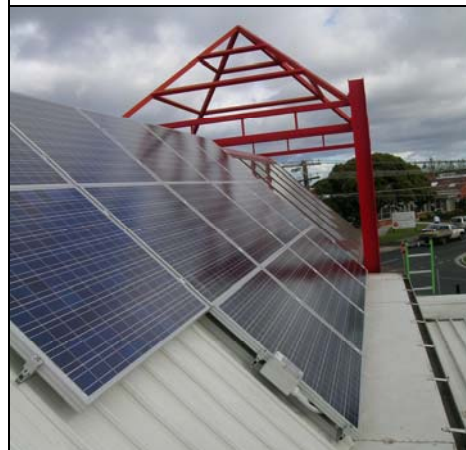
PV Panels on the roof
