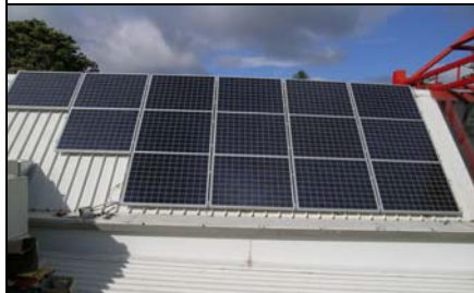
Photovoltaic panels on the roof
