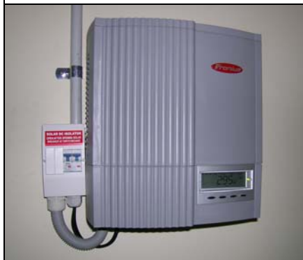
Inverter (located inside the building)
