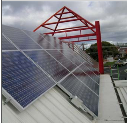
PV Panels on the roof
