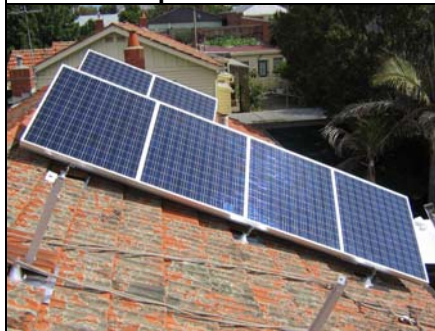
PV panels on roof
