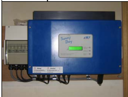
GI inverter in garage
