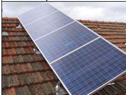
PV panels on roof
