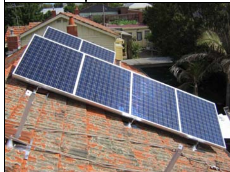
PV panels on roof
