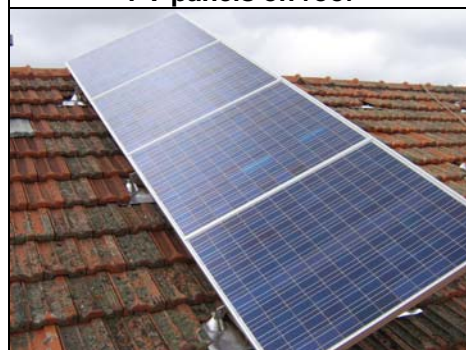
PV panels on roof
