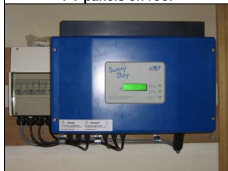
GI inverter in garage
