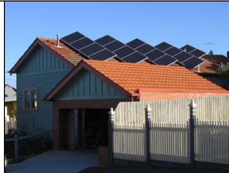
PV panels on roof
