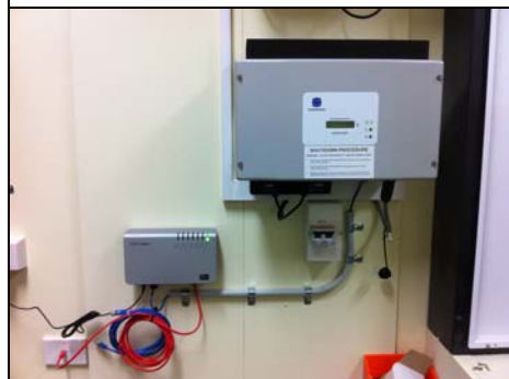
WebBox (left) and Inverter
