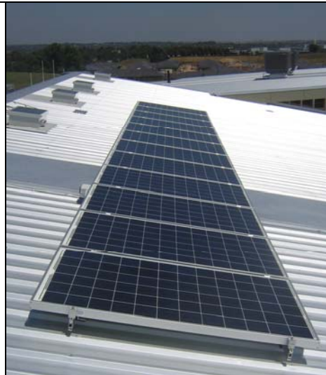
PV Panels on Roof
