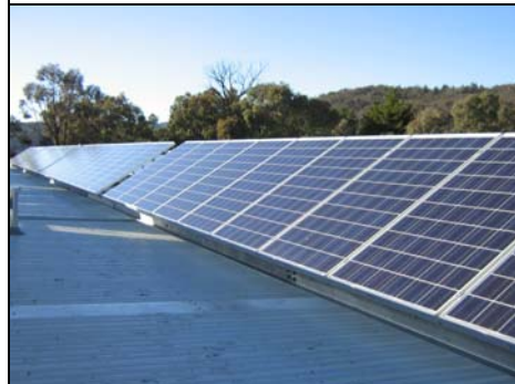
PV Panels on Roof
