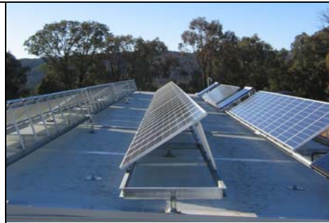
PV Panels on Roof
