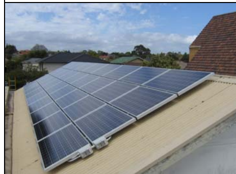
PV Panels on Roof
