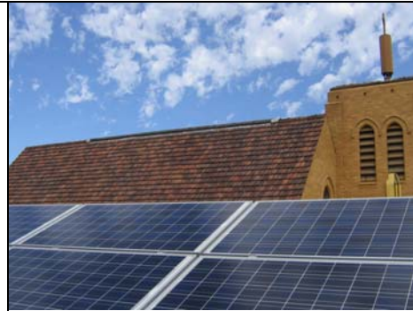
PV Panels on Roof
