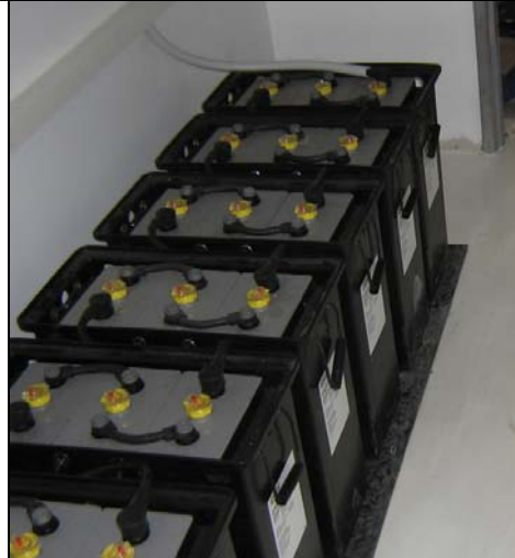
Batteries in leak-proof containers in ventilated room
