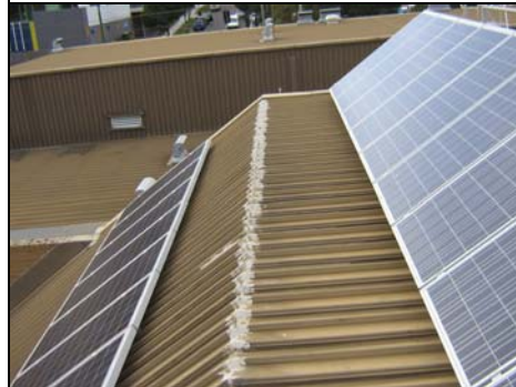
PV Panels on Roof
