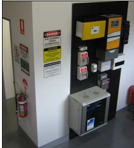
Battery Room, Control Panel, Safety Signage and Equipment
