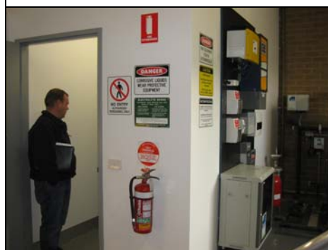
Dedicated Battery Room and Control Equipment
