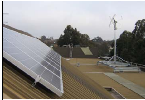
PV Panels & Wind Generator
