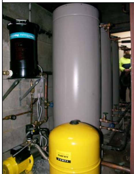
The pumps & storage tanks.
