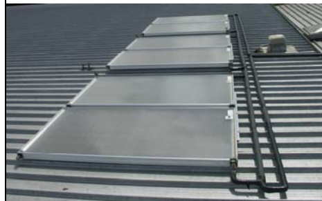
The solar hot water panels.
