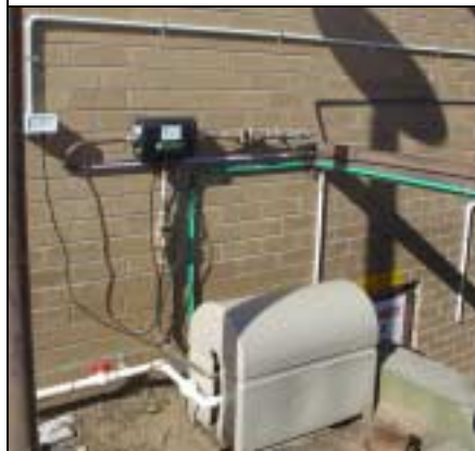
Rainbank & Pump Housing
