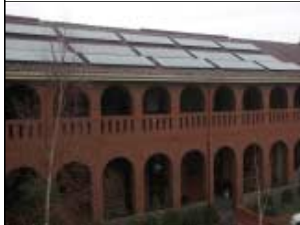
Roof Mounted PV Panels
