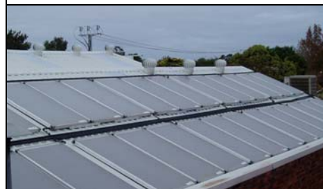
Solar Thermal Panels
