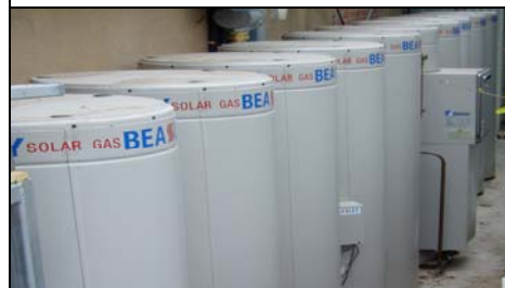
Thermal Storage Tanks
