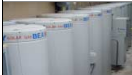
Thermal Storage Tanks
