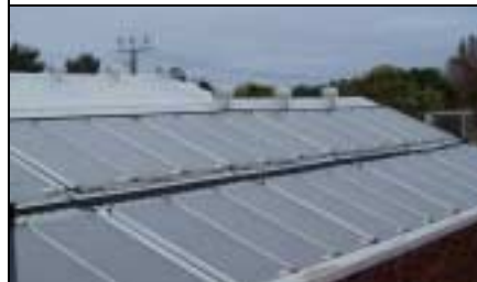
Solar Thermal Panels
