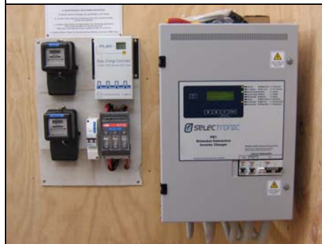
Controls and Inverter/Charger
