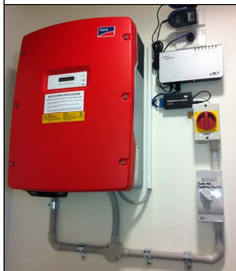
Inverter and Isolation Switches
