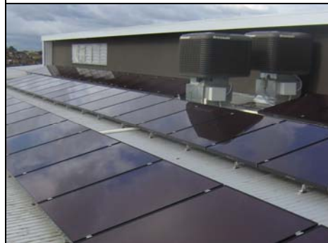
PV Panels on Roof
