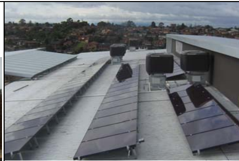
PV Panels on Roof
