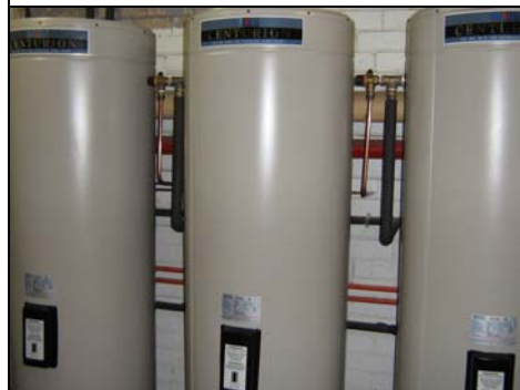
Stainless steel solar storage tanks
