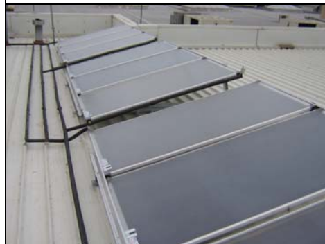
Solar Hot Water panels on the roof
