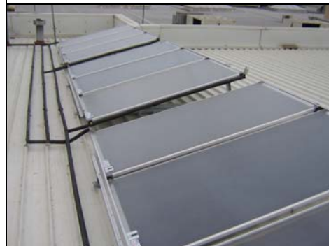
Solar Hot Water panels on the roof
