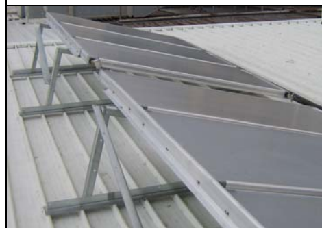
Solar Hot Water panels on the roof showing mounting frames
