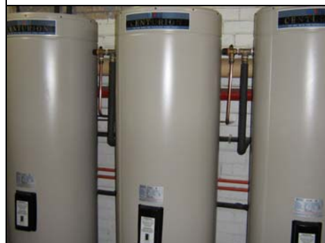
Stainless steel solar storage tanks
