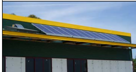
The PV panels on the eave
