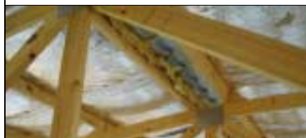
Foil and bulk roof insulation
