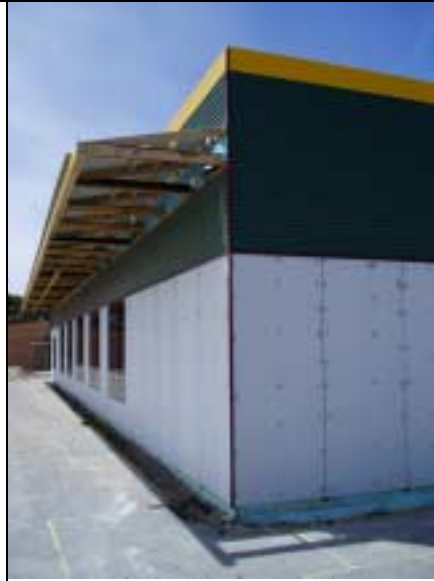
Reverse Brick Veneer and the Solar Eave – Note the shadow on 25 th Dec.
