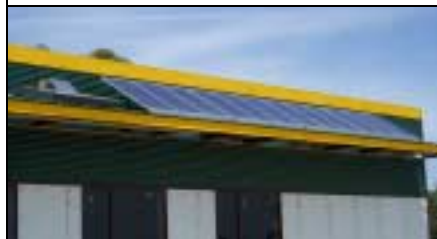
The PV panels on the eave
