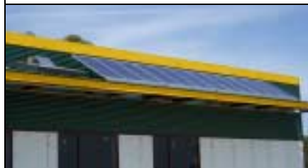
The PV panels on the eave
