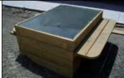
Observation window for the underground water storage
