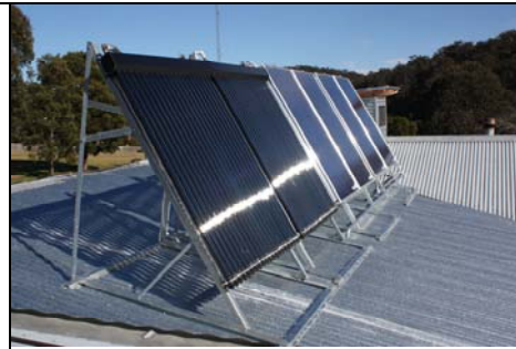
SHW Panels on Roof
