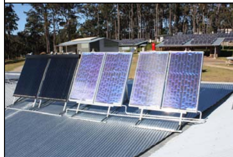
SHW Panels on Roof
