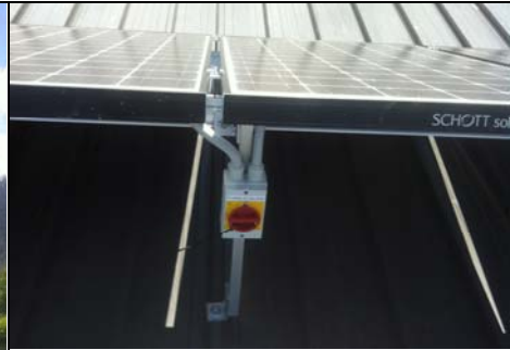
Rooftop DC Isolation Switch
