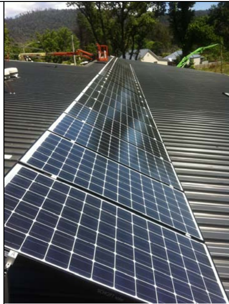
PV Panels on Roof
