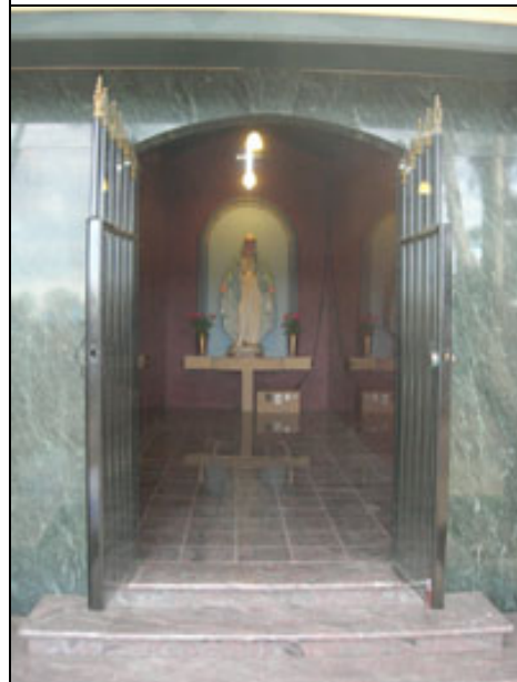
Lighting and Battery/Control Box inside the Mausoleum
