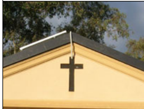
PV Cables through the Cross
