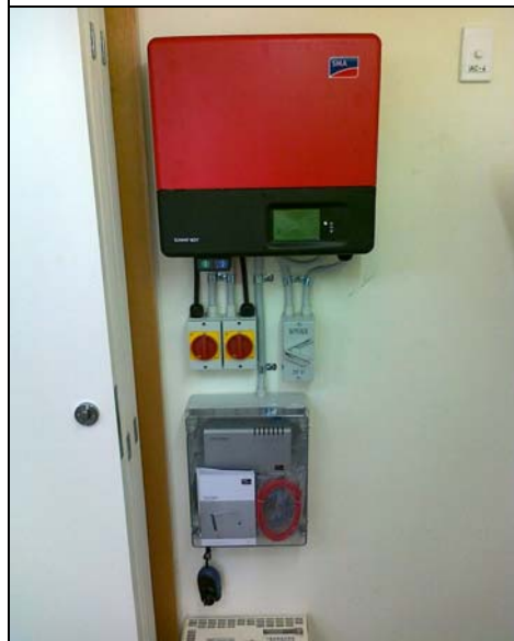
Inverter and Isolation Switches
