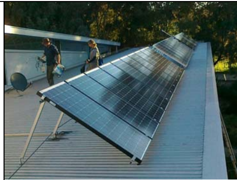
PV Panels on Roof
