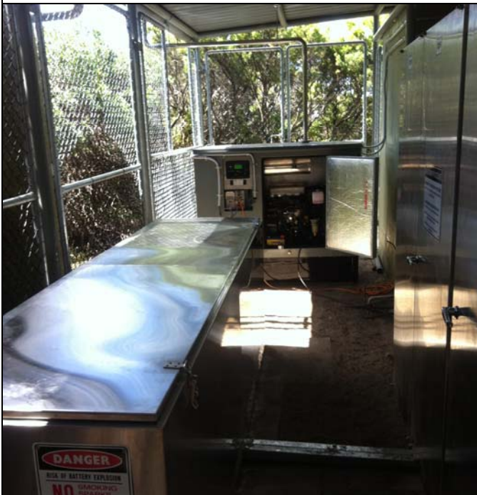
Control Room – Battery Bank on left, Inverter Cabinet at right, Generator at the back
