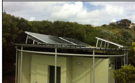
PV Panels on Roof
