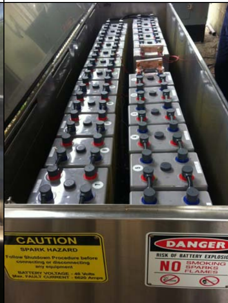
Battery Bank with battery cabinet lid open. Note the safety signage.
