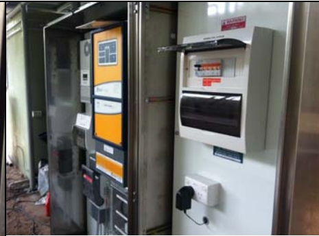
Inverter Cabinet and Fuses
