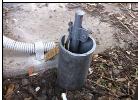
Detail of Earthing
