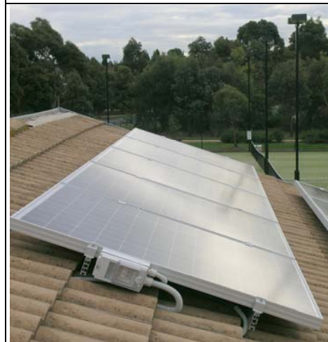
Detail of PV Bank
