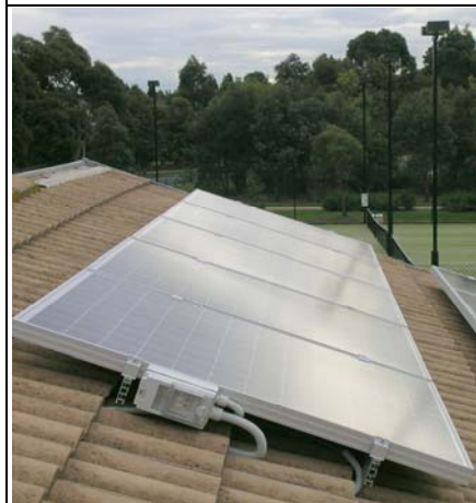
Detail of PV Bank
