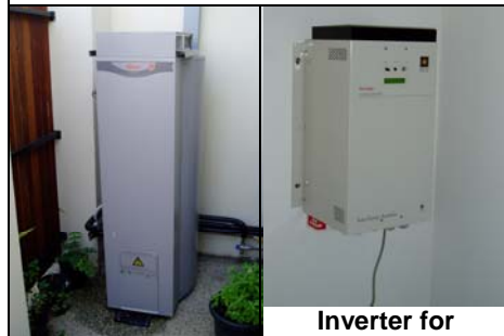
Solar hot water storage tank
