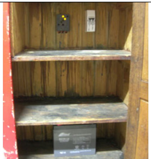
Existing Cupboard Housing Battery and Controls
