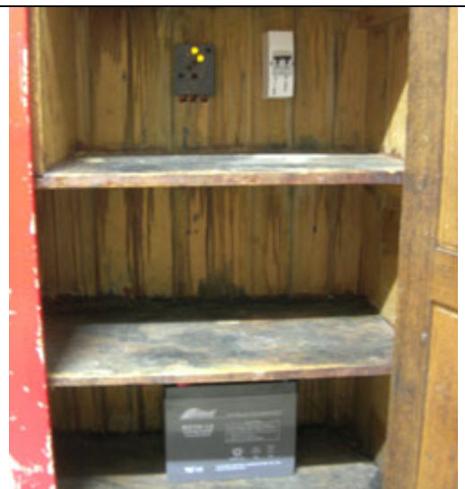
Existing Cupboard Housing Battery and Controls
