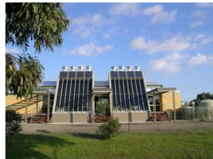
Eight 160W mounted to top of Solar Chimney
