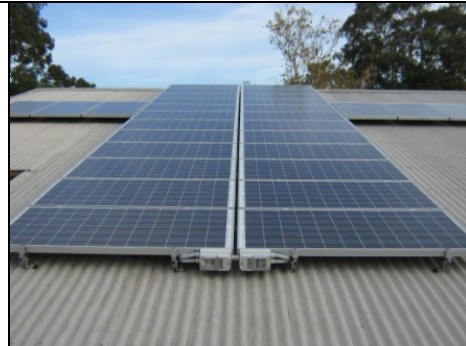
PV Panels on Roof
