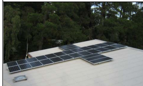
PV Panels on Roof
