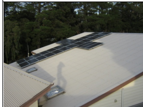
PV Panels on Roof
