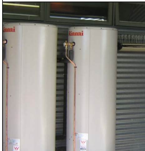
Hot Water Storage Tanks
