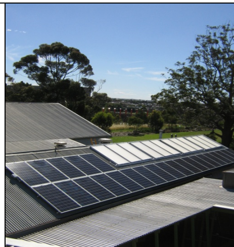
PV and SHW Panels
