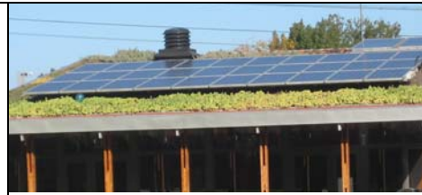
PV Panels on Roof
