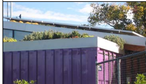
Edge of PV Panels on Green Roof
