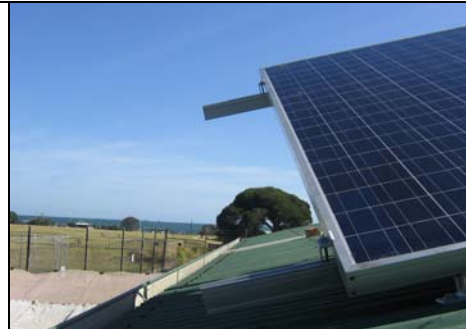
PV panel on roof
