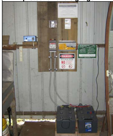
Sealed gel batteries
