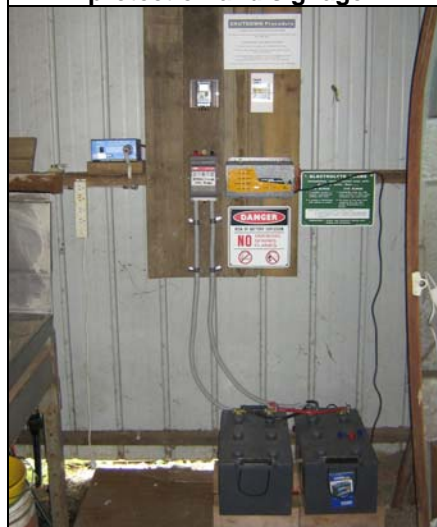
Sealed gel batteries
