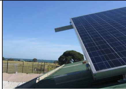
PV panel on roof
