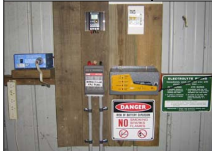
Inverter (blue box), solar regulator, battery charger, fuse protection and signage
