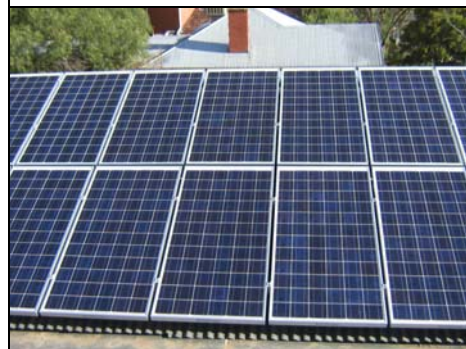
PV Panels on Roof
