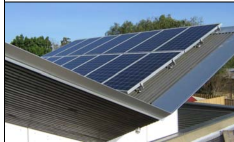
PV Panels on Roof
