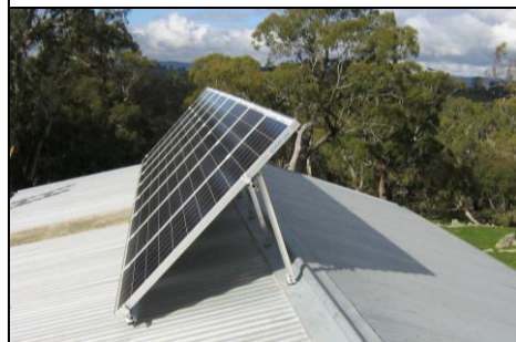
PV Panels on the Shed Roof
