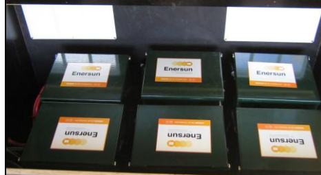
Batteries (lids closed)
