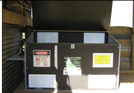
Battery Box with Signage
