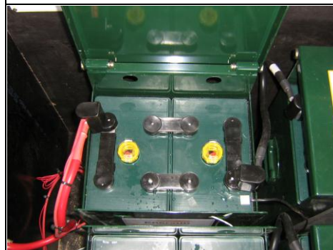
Detail of Battery (lid open)
