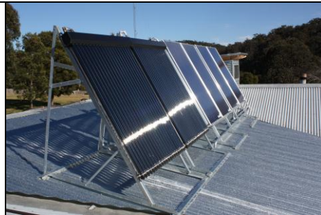
SHW Panels on Roof
