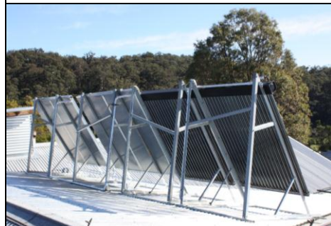
Rear of SHW Panels on Roof
