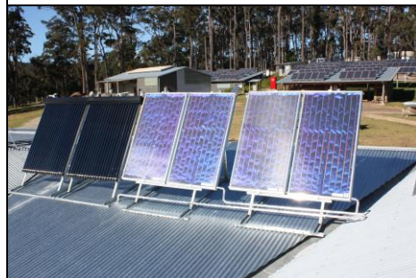
SHW Panels on Roof
