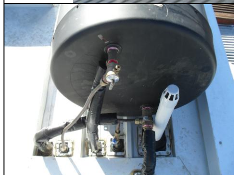
Detail of Storage Tank
