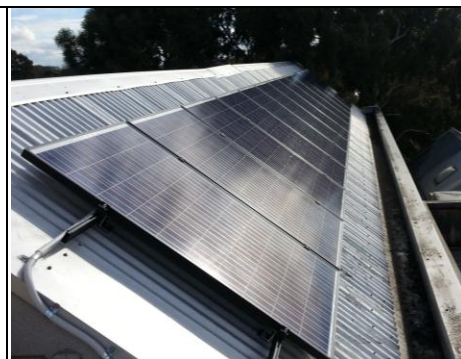
PV Panels on Roof
