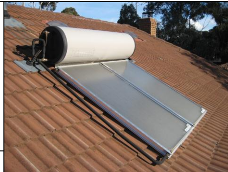
SHW system on roof
