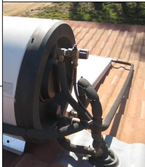
Detail of insulated pipes, valves and roof penetration
