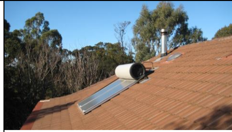
Solar hot water system (with wood stove flue above it)
