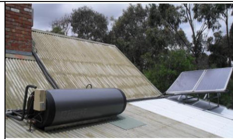
SHW Tank & Panels on Roof
