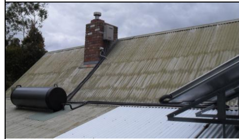
Solar Panels, Tank & Gas Booster
