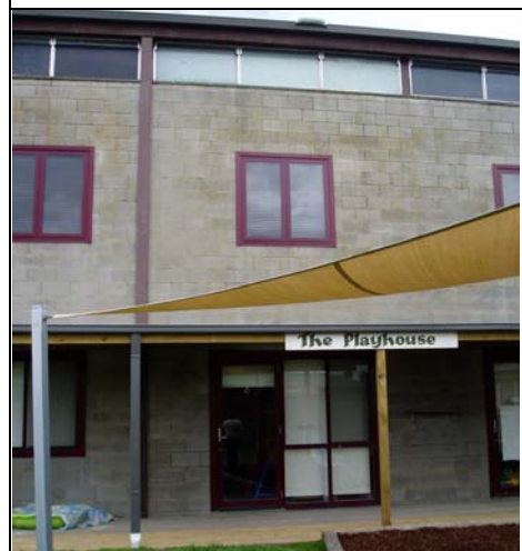
Protection needed from the sun on the north-facing windows & walls
