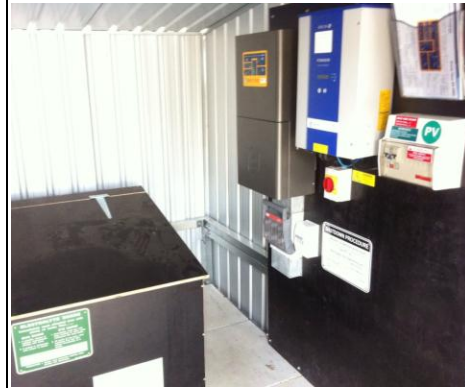
Inside Control Shed
