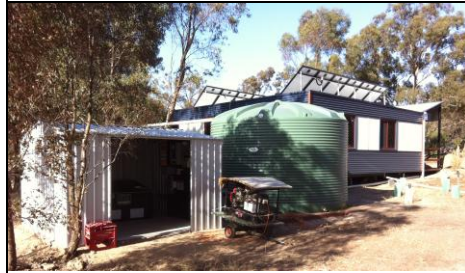
Control Shed & Rear of PV Panels
