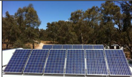
PV Panels on Roof
