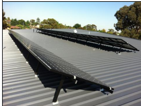
Rear of PV Panels
