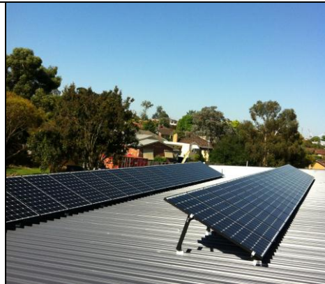
PV Panels on Roof
